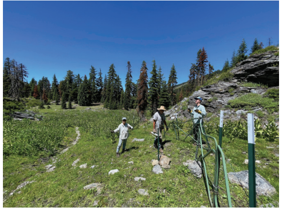
KS Wild volunteers repairing a fence in Alex Hole Meadow. Photo credit: Haleigh Martin
